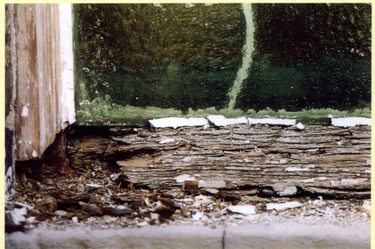
3. Window adversely affected by wood decay.
